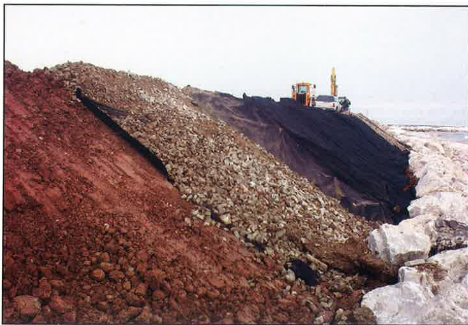
The next step of a buried revetment is completely conventional. Fabric, bedding stone, then armor stone are placed in succession.
