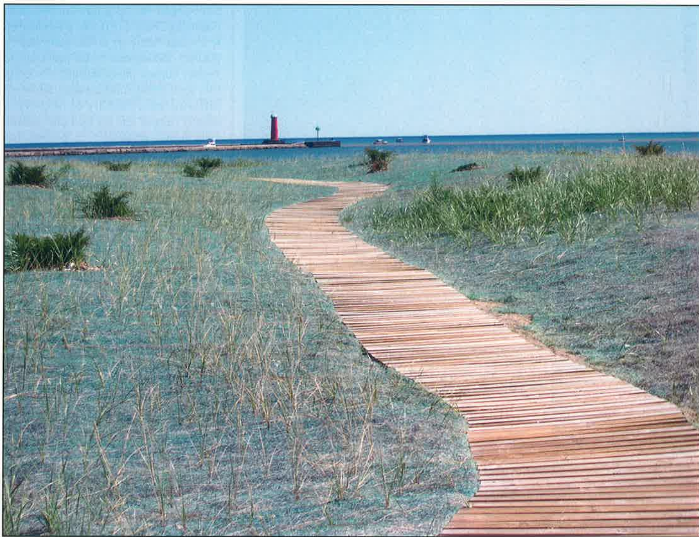
Planted dune grass is an important component of the buried revetment system.
