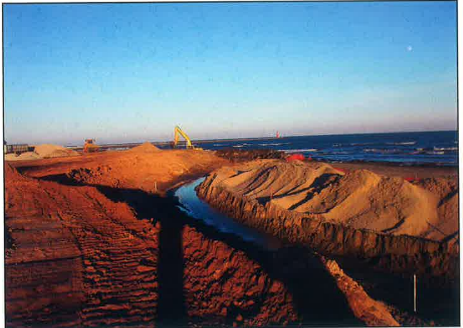
The first step in construction of a buried revetment is excavation for its toe, with the sand placed outboard to later become a fore-dune.
