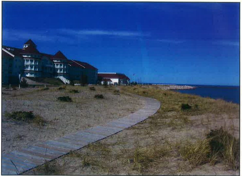
Dune grass planted over the “buried” revetment (invisible but just to the right of the boardwalk) takes hold in just one year.
